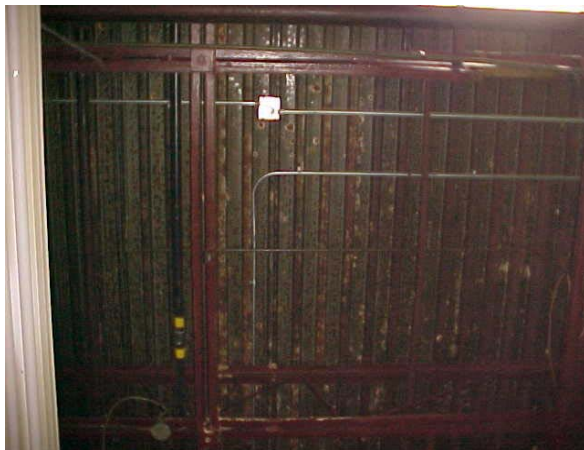
Roof Deck Corrosion
