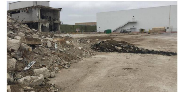
Demolition under way at the north side of the former Six Flags Mall, clearing space for an industrial complex.
